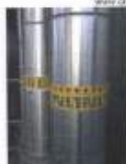
Pipes carrying biogas
